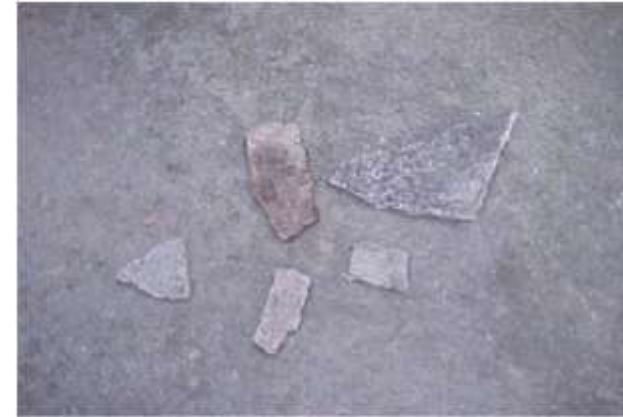
Photo 3 – Flat Asbestos Cement sheet fragments
